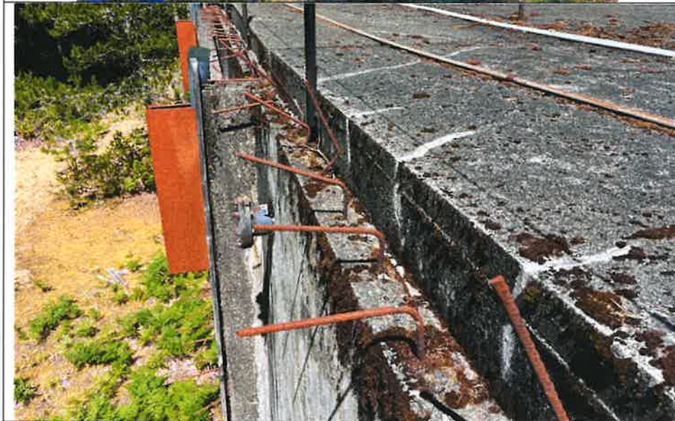
Photo 6 - A view of the exposed rebar on the south side of the water tank.
