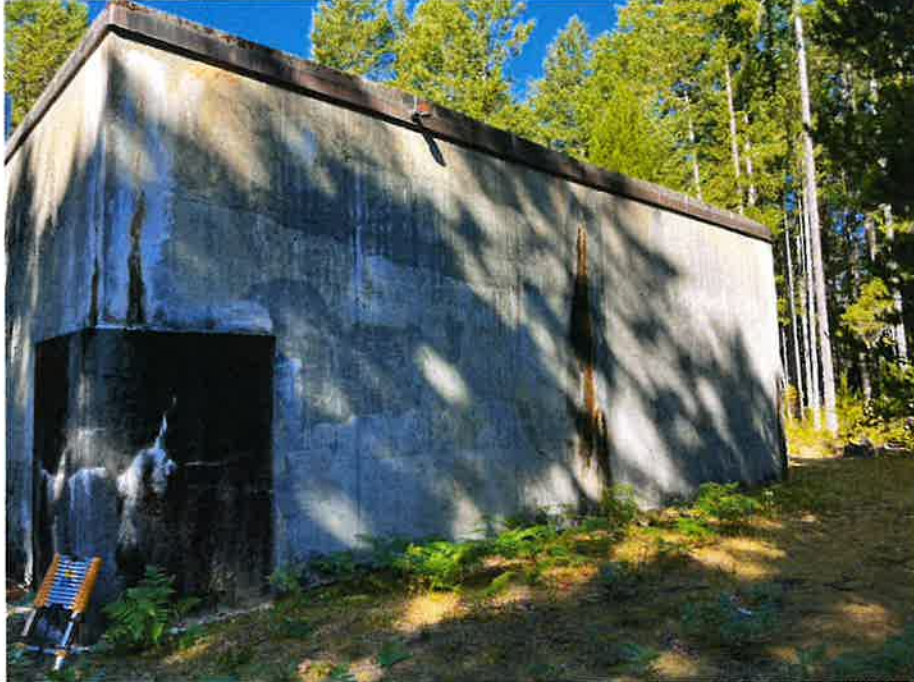
Photo 3 – A view of the north side of the holding tank. Note the vertical cracks near the corners as well as in the center.
