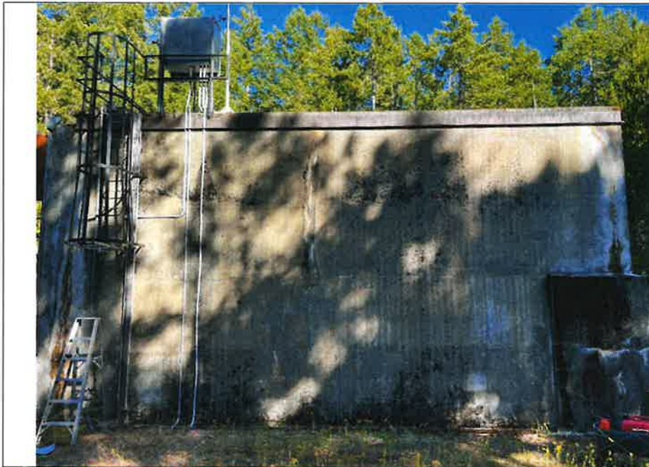
Photo 1 – A view of east side of the water tank. Note the vertical cracks near the corners as well as in the center.
