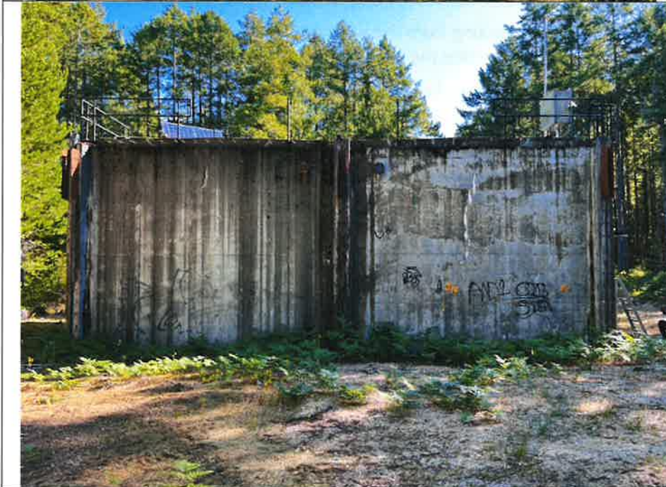
Photo 2 – A view of the south side of the holding tank. Note the vertical cracks near the corners as well as in the centers.
