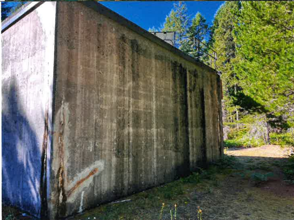
Photo 4 – A view of gauge the west side of the holding tank. Note the vertical cracks near the corners.
