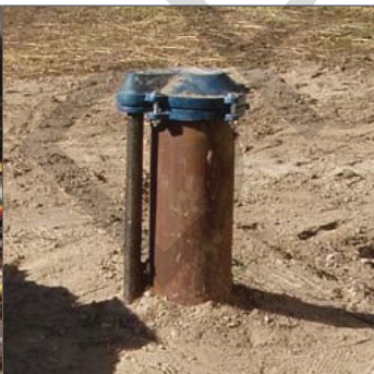
FIGURE 6 Well fitted with pitless adapter, cap has space for wiring
