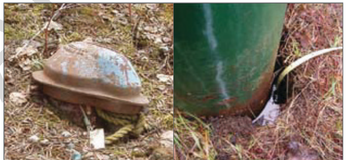
FIGURE 1 Well casing stickup less than 30 cm (1ft) from the ground surface
