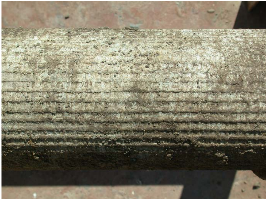
Figure 2: Close-up view of AC pipe Sample X-87 (Lot 10, Shoreline Drive) in the as-received condition, showing adhered dirt and sand and the heavy waffle pattern on the sample external diameter surface.
